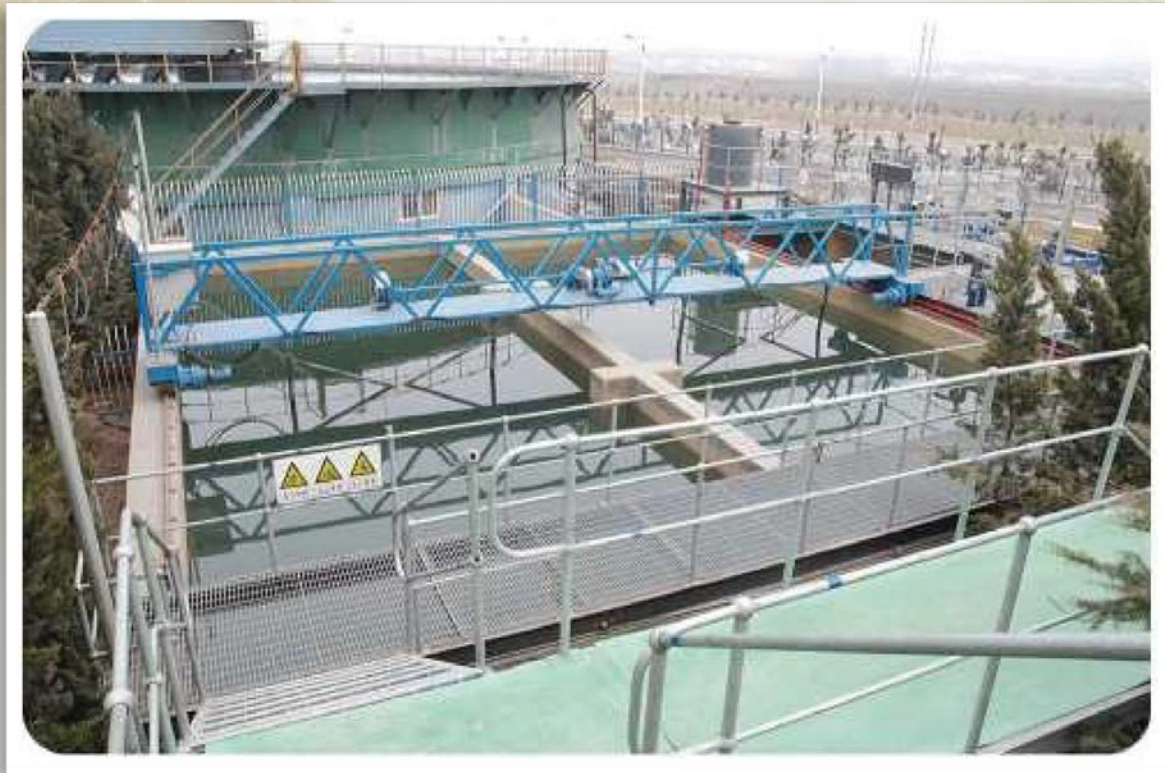
The picture shows the water purification treatment system of the Jinchiling Gold Mine
