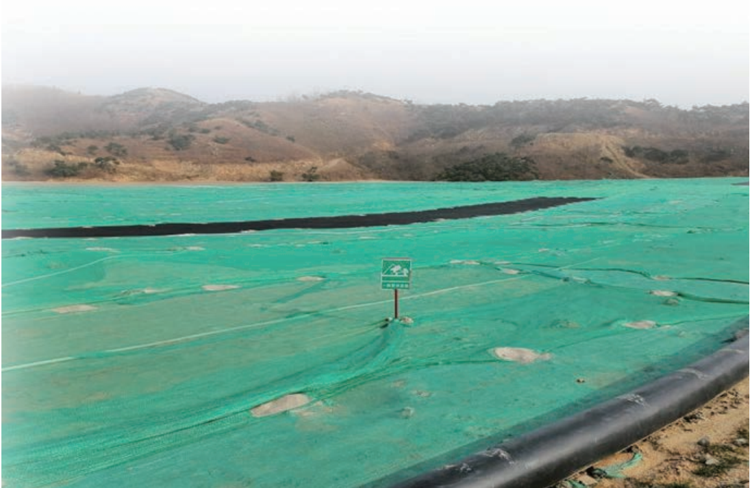
Dust control netting on dry beach of tailing pond can effectively eliminate dust
