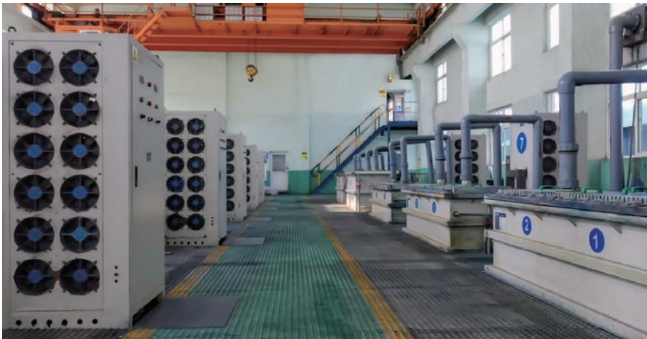
Jinchiling Gold Mine Water Treatment System
